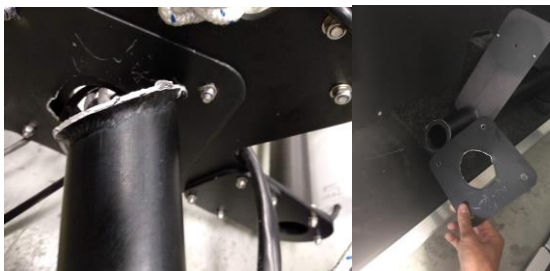
Figure 25: Damage to the Antenna Mast
